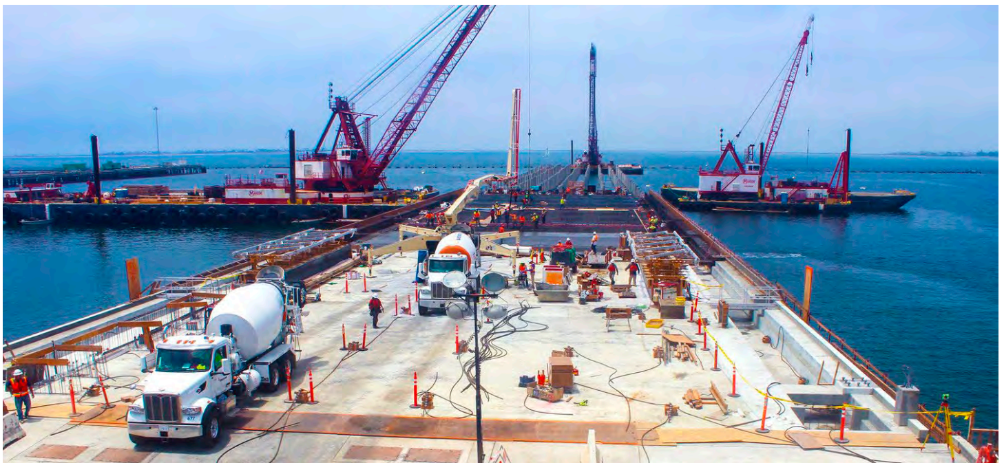
Figure 1: Manson project crews working at the P-443 Pier 6 Replacement project site with multiple concurrent phases of work occurring at NBSD, CA (2021-2023).
